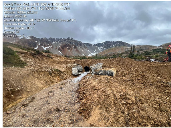
Plate 006: Photo KW005 Stream Habitat of 900 proposed at site KN001. Gradient and velocity barrier site FB1.
