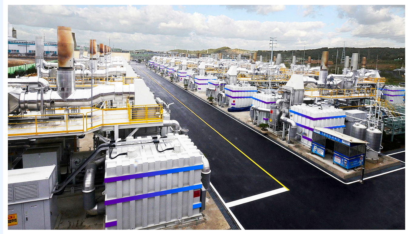
Gyeonggi Green Energy - 58.8 MW fuel cell park provides power and heat to local homes.
