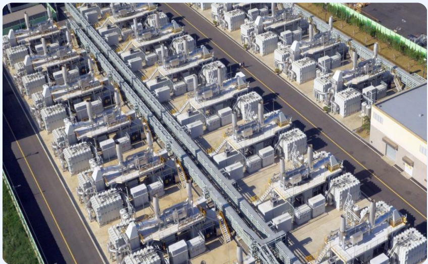
GGE, South Korea - one of the largest fuel cell parks in the world, established in 2013
