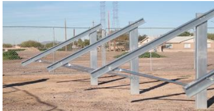
Original deployment of ground-mount solar
