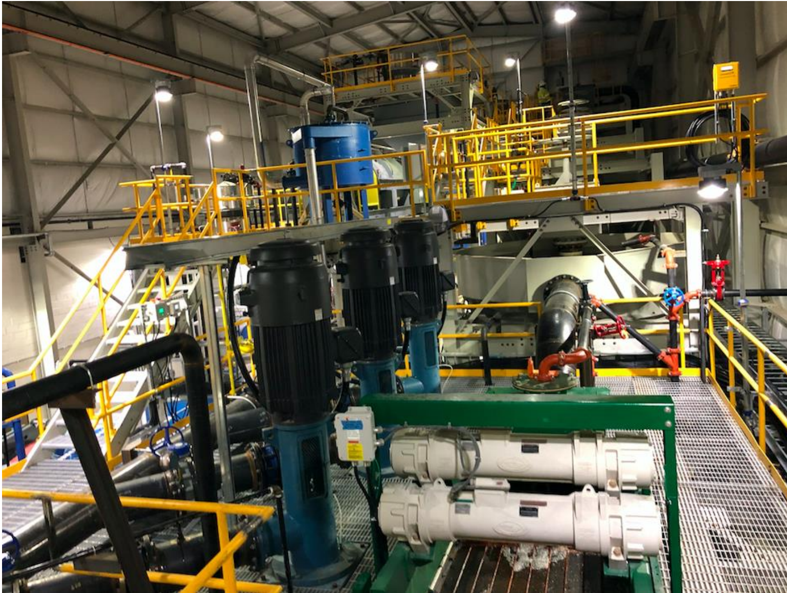
Solution Transfer Pumping System
