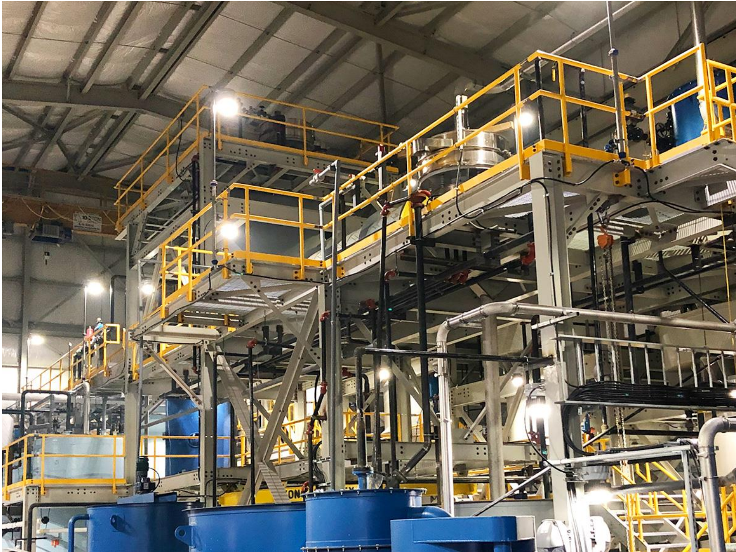
Inside Mechanically Complete Process Plant
