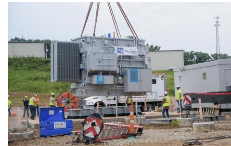
In Franklin County, crews installed a new, made in Missouri substation transformer to support reliability for over 2,700 homes and businesses.
