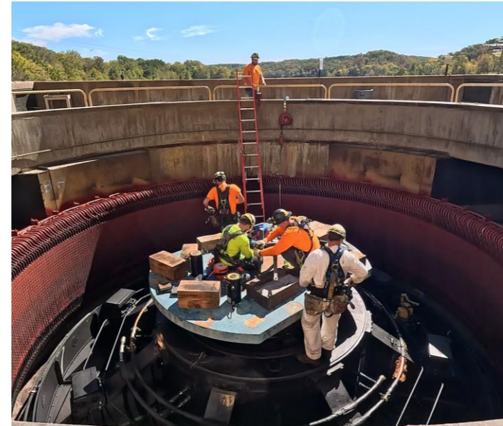
Ameren Missouri replacing the last of the original turbines (circa 1931) at Osage Energy Center with stronger, more flexible erosion-resistant steel runners.
