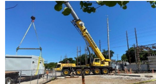
Upgraded Sparks Substation energized in 2022 ~3,800 residential and business customers to benefit
