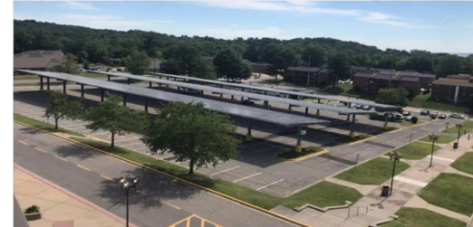
Cape Girardeau Renewable Energy Center in service July 2022 1.2 MW facility
