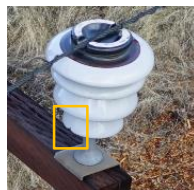
Cracked Insulator visible in zoomed image
