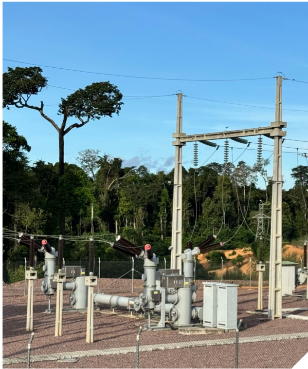
Electrical substation at TZ Mine
