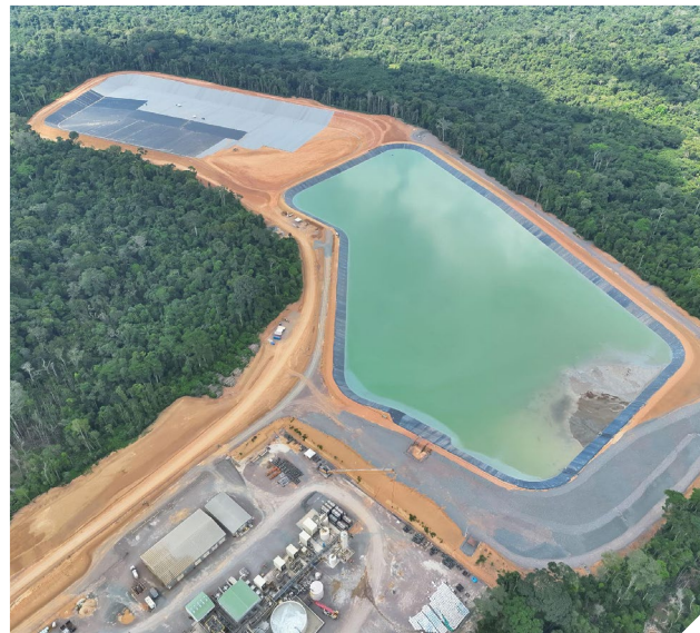
Cyanide/CIL Tailings Storage Facility (CTSF) at TZ Mine
