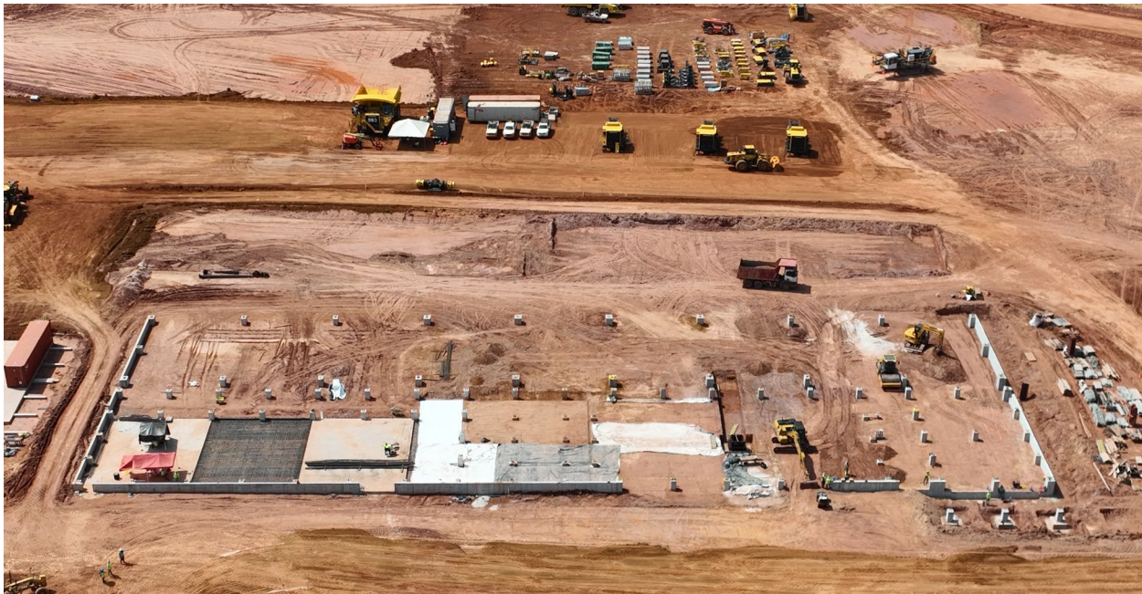
Photo: Foundations for the Mine Maintenance Facility are progressing, with completion targeted for Q2 2026 with steel structure erection to follow.
