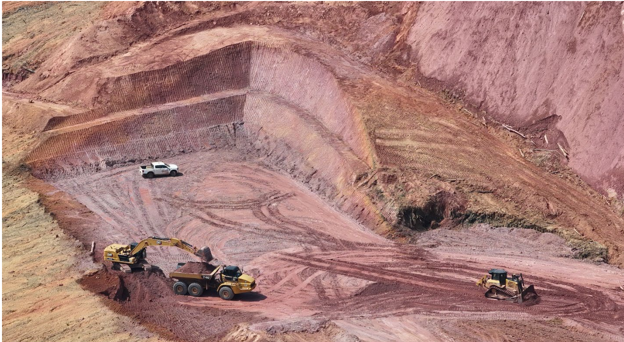
Photo: Mass excavation for the primary crusher is complete, and the area is ready for concrete works to commence.
