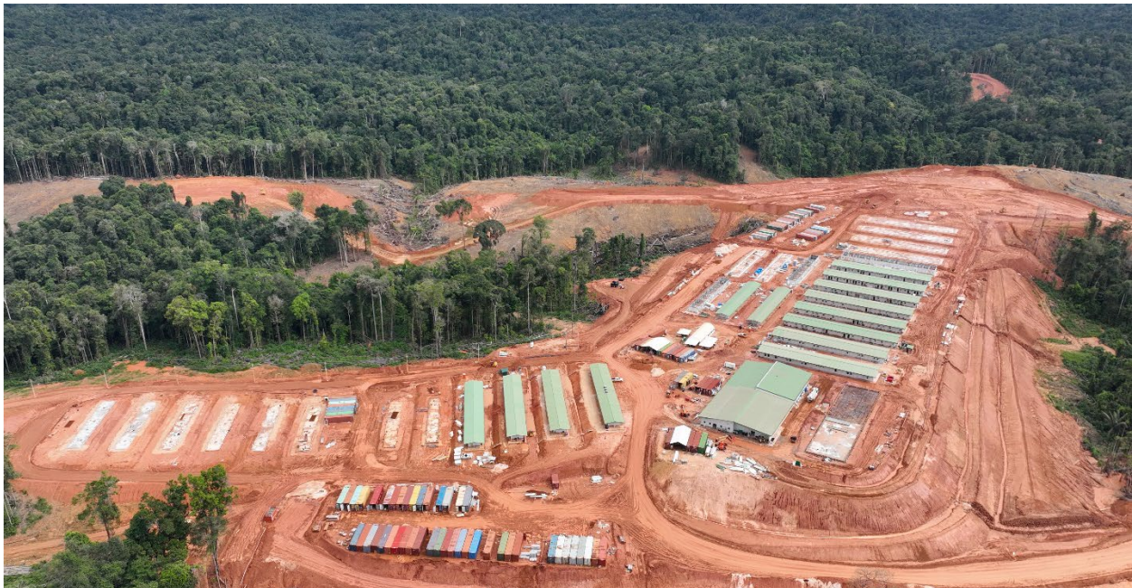
Photo: Camp infrastructure continues to expand, with additional dormitories being delivered through 2026. A large central building housing the kitchen and mess hall is scheduled to be operational in the second quarter.
