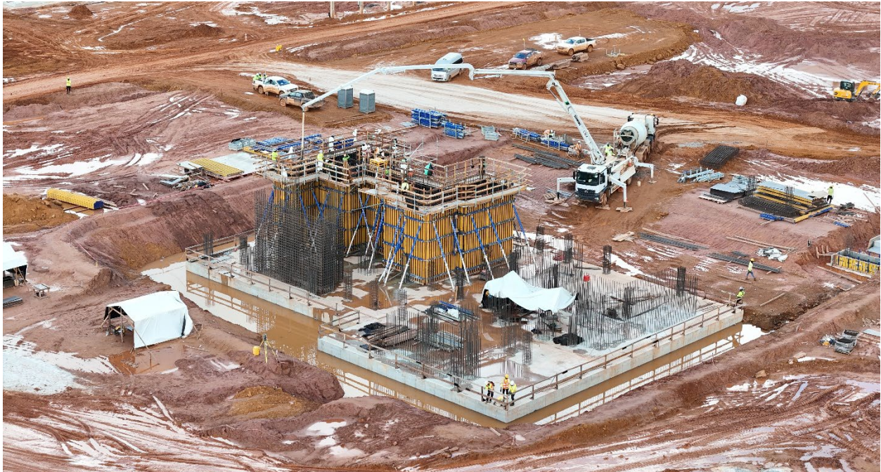
Photo: Concrete work in the grinding area is progressing, with formwork installation and rebar placement for the SAG mill piers well advanced. The ball mill foundation can be seen on the right.
