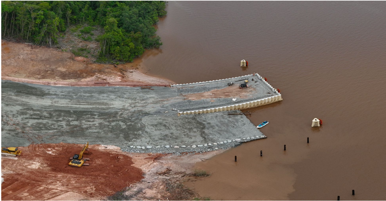
Photo: Our newly commissioned wharf was completed in mid-April and is now ready to accommodate barge landings for the unloading of heavy equipment, as well as construction and mining materials.
