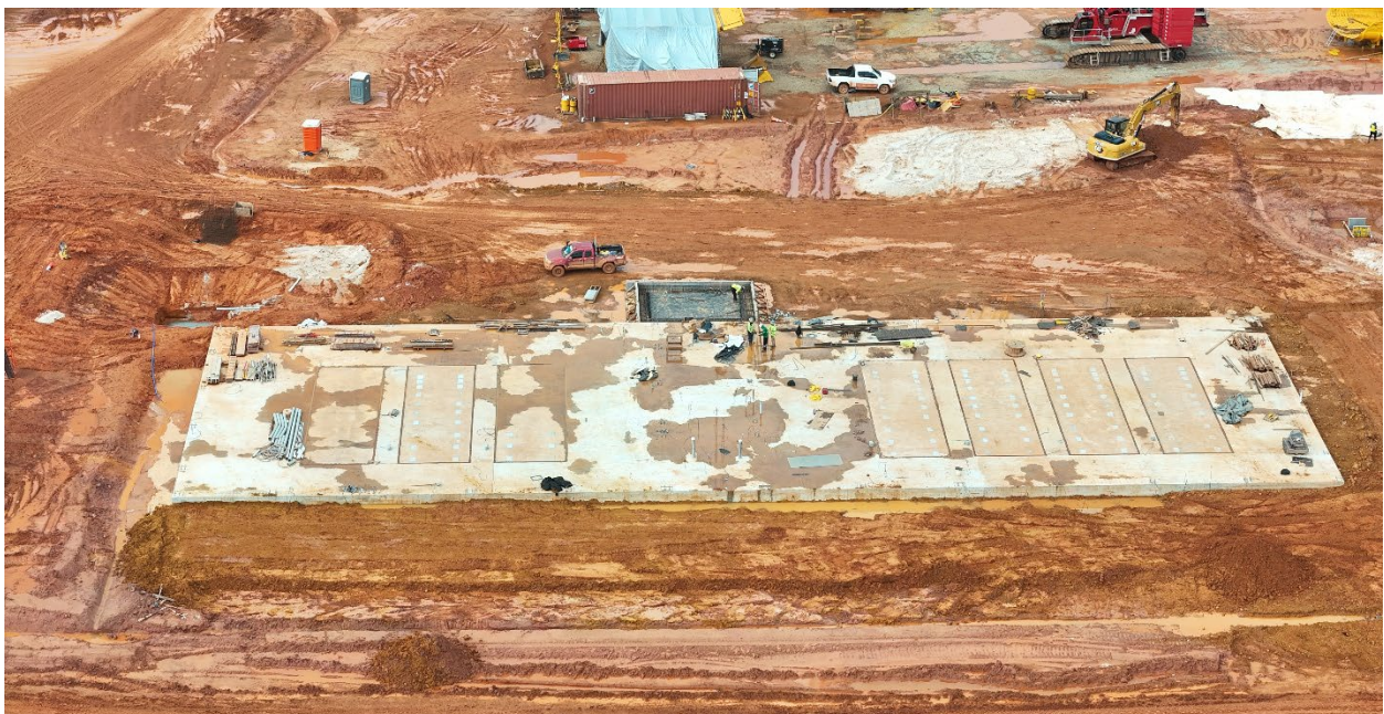
Photo: The power plant foundation has reached a major milestone, with the concrete pour completed and the site ready to receive the generators.
