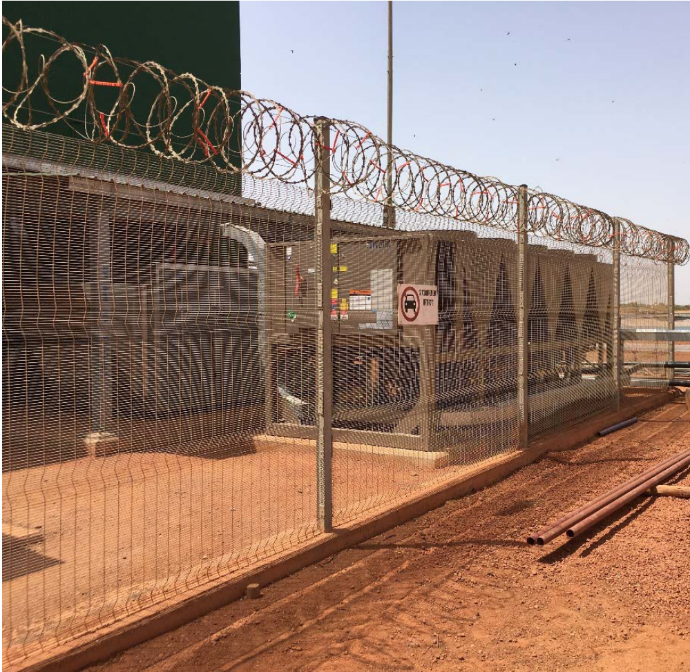
Gold Room HVAC
