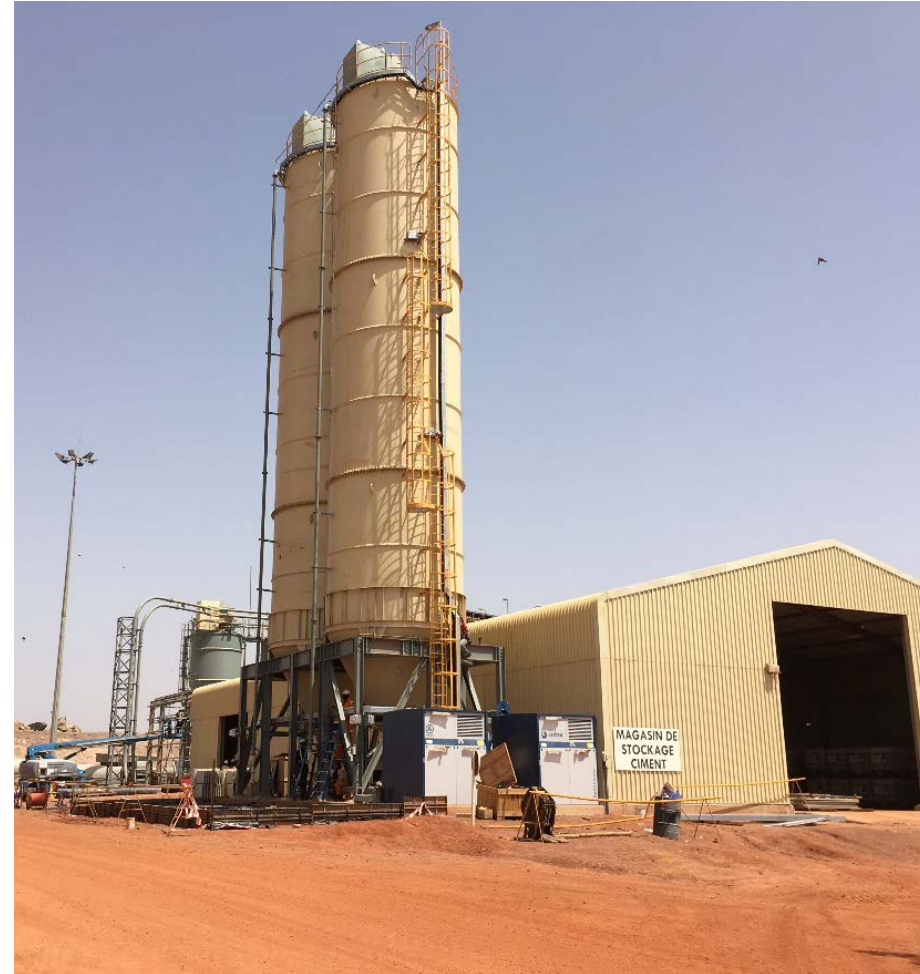
Cement Silo System
