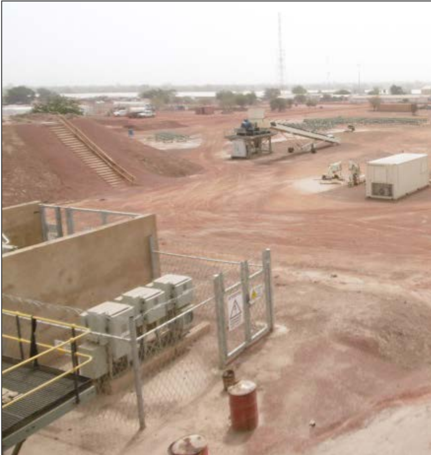
Feed Preparation Circuit - Before
